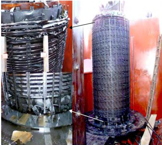
Figure B.19 – Frequency response of an LV winding before and after axial collapse due to clamping failure with a photograph of the damage [8]
