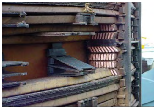
Figure B.20 – Frequency response of a tap winding with conductor tilting with a photograph of the damage [1]
