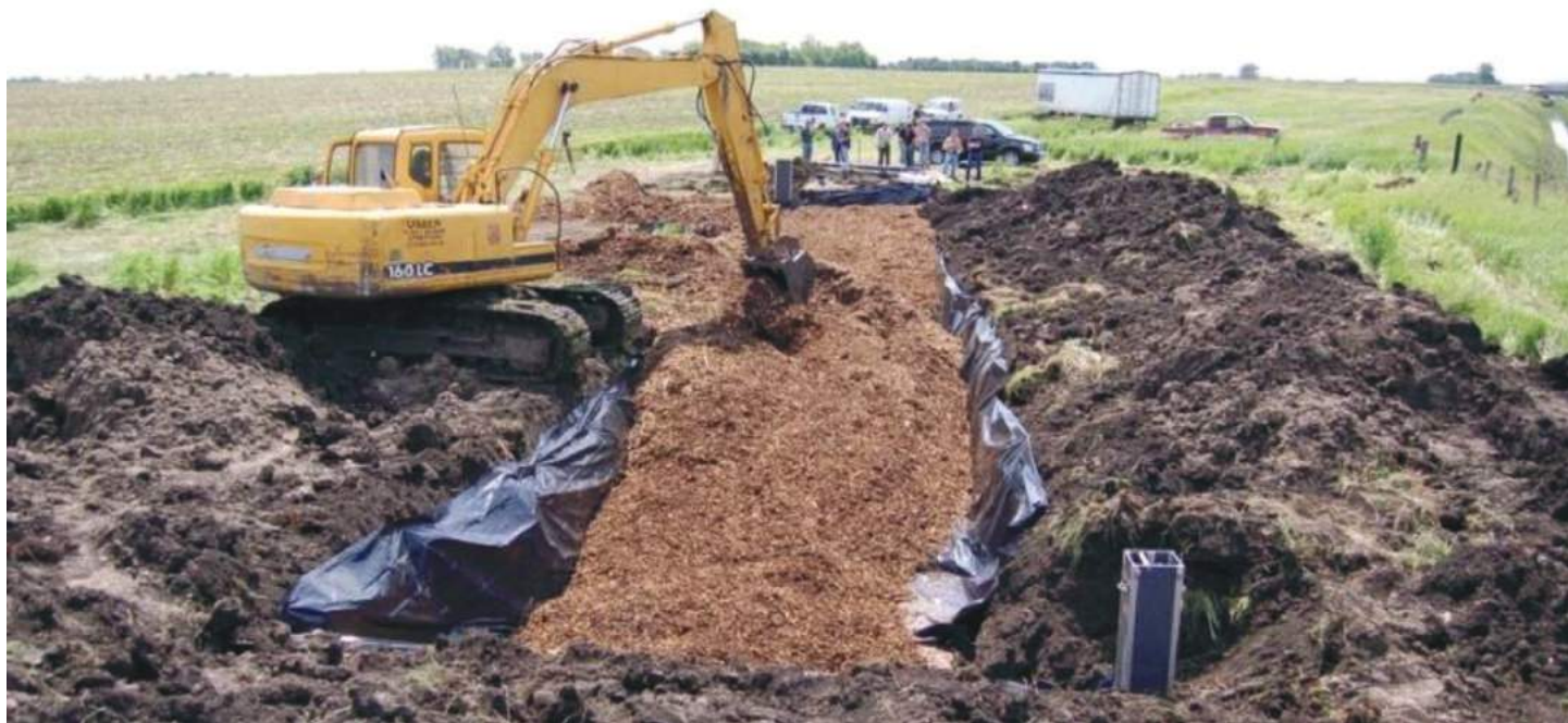
Figure 24: Bioreactor during construction (courtesy of the Iowa Soybean Association Environmental Programs and Services; from Christianson and Helmers, 2011).
