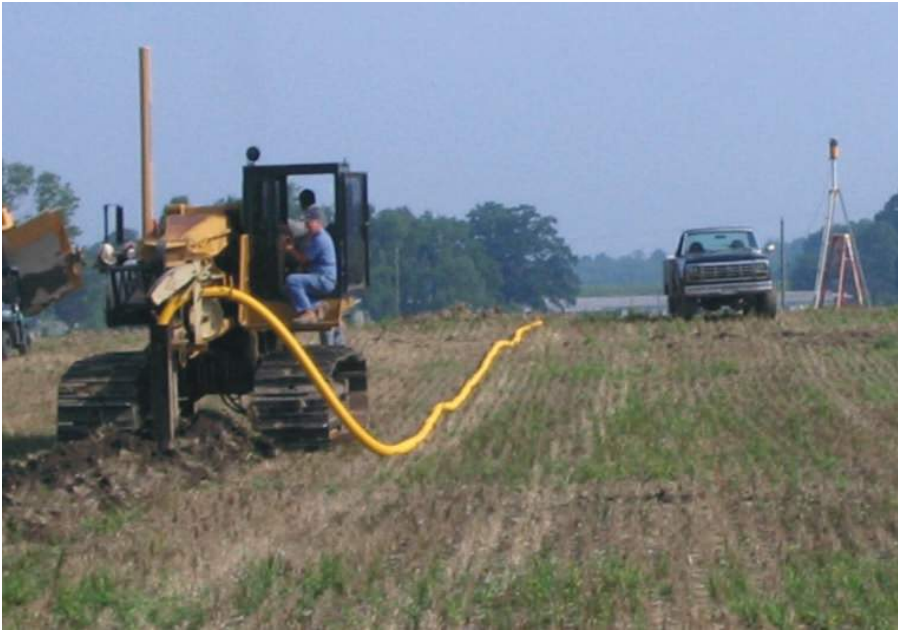
Figure 3: A drain plow installing corrugated plastic tubing known as tile drainage. Vertical placement in the soil is guided by a laser system or GPS to ensure consistent grade.
