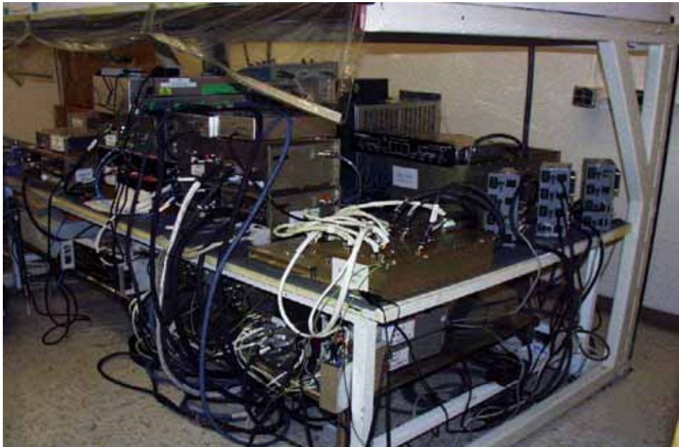
Figure 4-13. The Integrated Test Facility (ITF) flight simulator hardware in a Clean Room at Lockheed Martin
