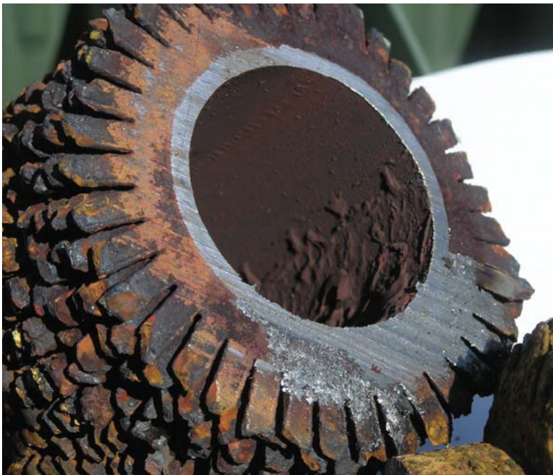
8. Leaky heaters. This HRSG feedwater heater tube was one of many failures that resulted from cold-end corrosion during cycling. There were numerous leaks at the
