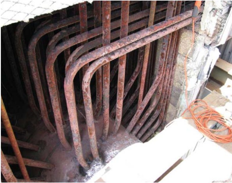
7. Inflexible headers. Reheater outlet header and tube-to-header weld fatigue damage at the end of the header is shown. The high-stress location is the short run of tubing where the tube cracked, due to low tube flexibility. The stress is a result of thermal loading and deflection during startup cycles. Courtesy: Intertek-Aptech
