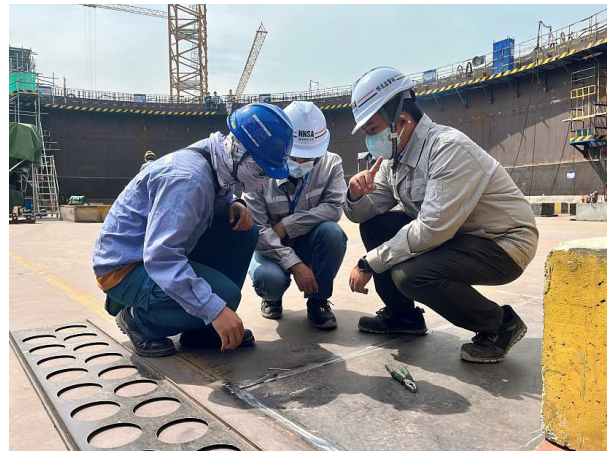
Figure 5. Quality supervision of submerged arc-welding of steel lining base plate welds of Tianwan NPP Unit 8
