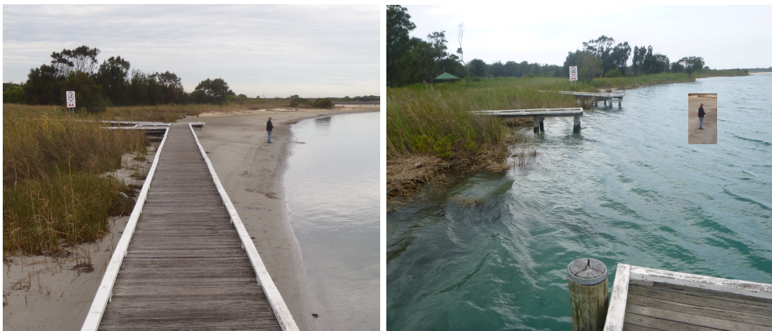
Figure 6: Shots of the northern entrance channel foreshore downstream of Windang Bridge taken on the 14-6-2012 (left) and 12-3-2015 (right), showing the loss of intertidal shoals and sections of boardwalk lost through scouring of the pilings.
