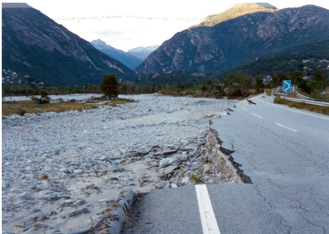
Figure 2.1. Destruction of the main highway from Milan to the Simplon pass (Switzerland) by floodwaters, Piemonte, Italy 13-16 October 2000
