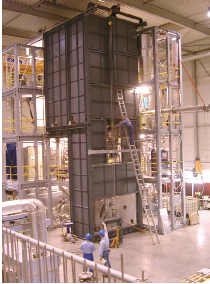
Figure 5: BTG 50 t/d rotating cone fast pyrolysis plant in Malaysia
