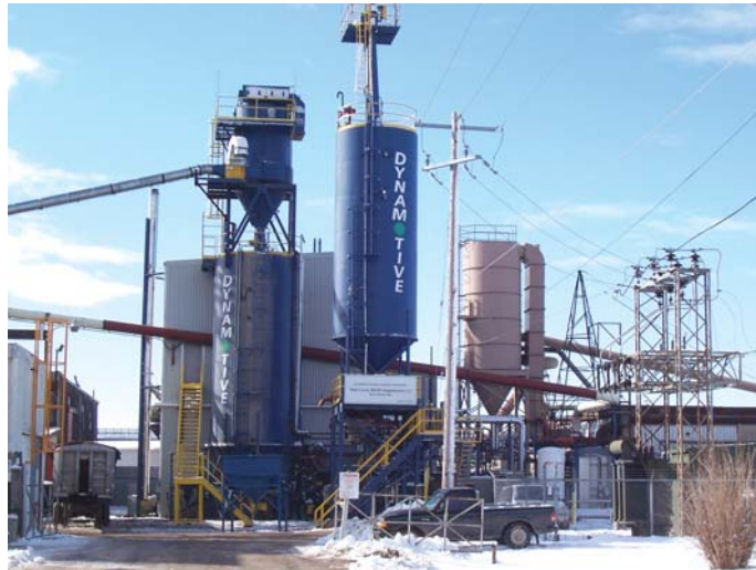
Figure 2: Dynamotive 100 t/d fluid bed fast pyrolysis plant in West Lorne, Ontario, Canada
