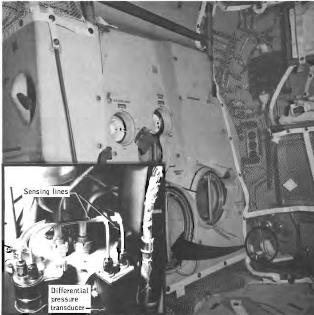
Figure 14-25.- Glycol pump sensing lines.
