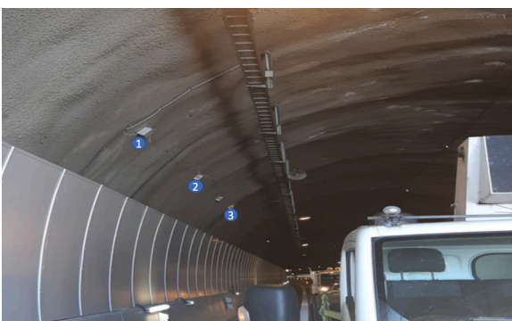
Fig. 6. Monitoring nodes installed in a Tunnel deployment of the architecture in Spain.
