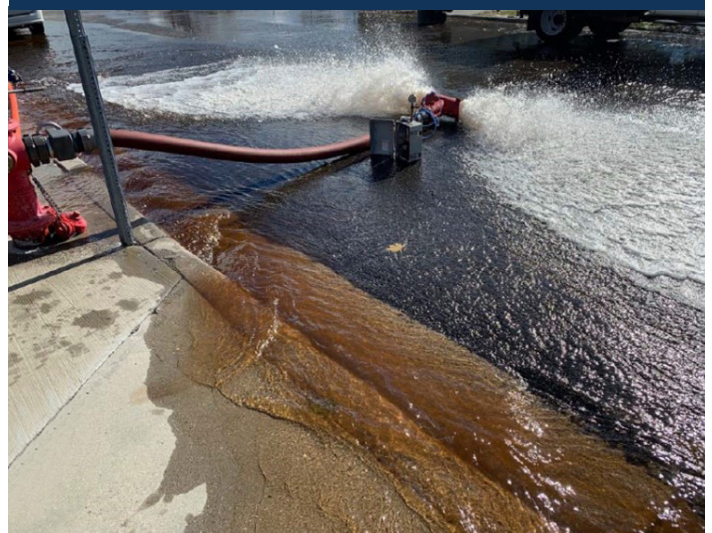
FIGURE 3: FLOW DISCHARGE THROUGH HOSE MONSTER
