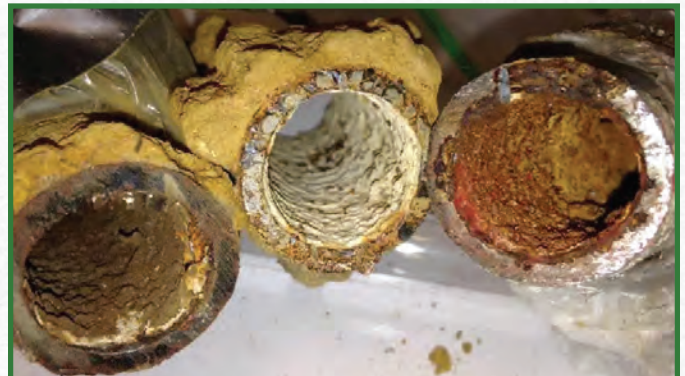
FIGURE A.25 : CORRODED IRON PIPE SAMPLES FROM FLINT, MI
