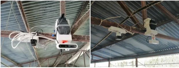
Fig. 2. Photos of the monitoring system.
