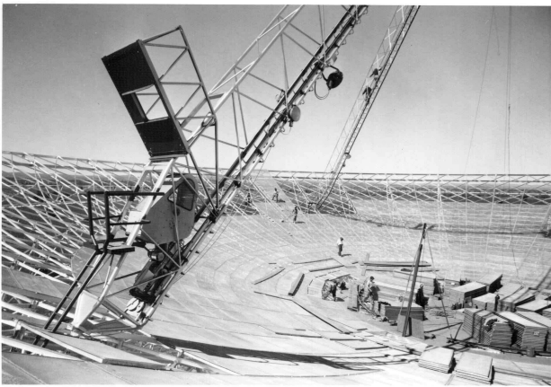
FIG. 13.— Over 1000 steel mesh panels were fitted to form the reflecting surface of the dish. The aerial cabin above can be reached via the small lift within the tripod leg.
