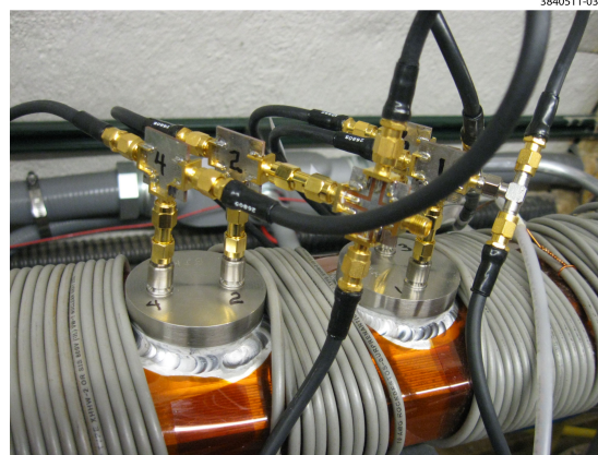
Figure 33. Photo of Shielded Pickups installed at 15E with the installed solenoid winding
