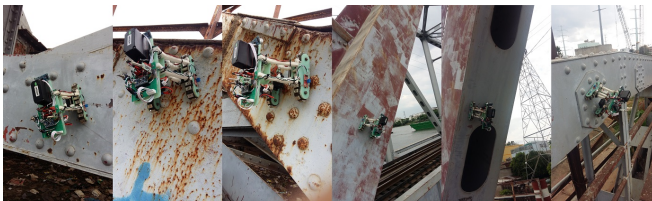
Fig. 17: Adhesion and climbing test on a rusty paint-coated steel bridge: flat structure with bolts/nuts. Video click here: https://ara.cse.unr.edu/?page_id=11
