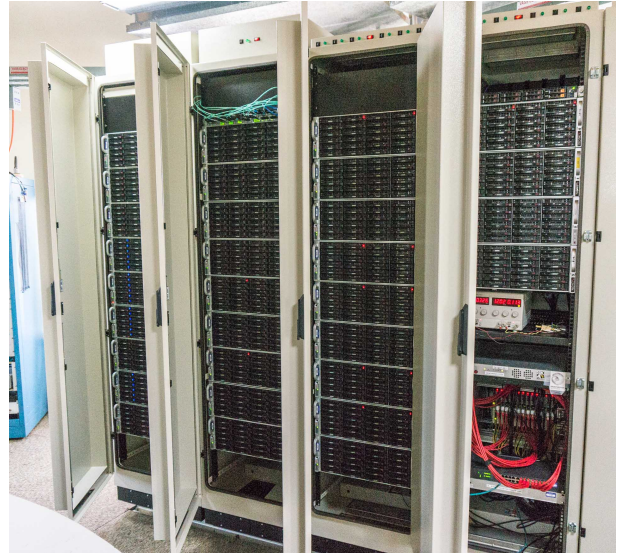
Figure 4. Rack front pic.
