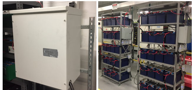
Figure 6: UEP battery system. (Left: battery rack. Right: inverter)
