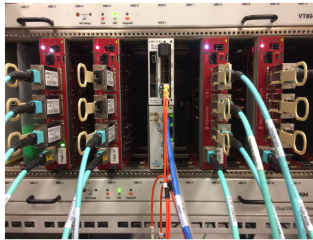
Figure 9. The demonstrator test system. The system was based on the CTP7 MicroTCA blade, used in the current CMS trigger. The system consisted of four CTP7s. Each CTP7 has 63 input and 48 output 10 Gb/s optical links.
