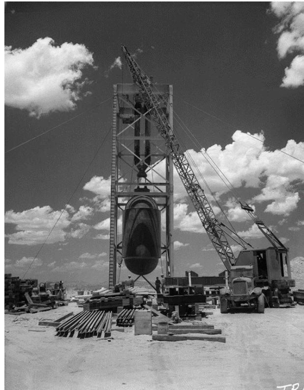
Figure 28. Jumbo suspended by a large block and tackle in the tower, circa summer 1945. Note the missing x-bracing where Jumbo was hoisted from horizontal at the base of the tower to vertical within the tower.
