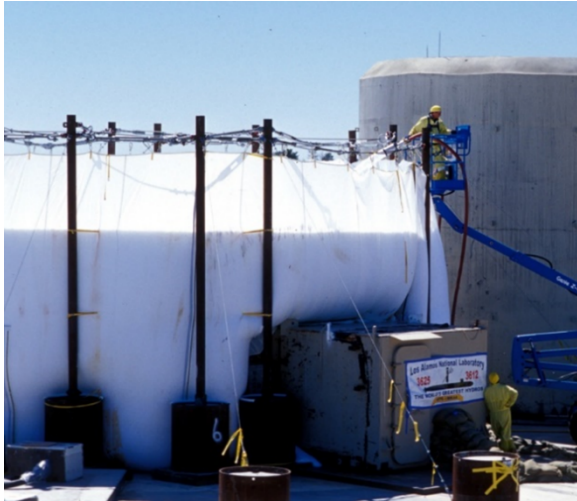
Figure 8. Filling a confinement “tent” with water-based foam prior to a hydrodynamic shot at DARHT. Foam shots were conducted from 2001-2005 before moving to vessels in 2006.
