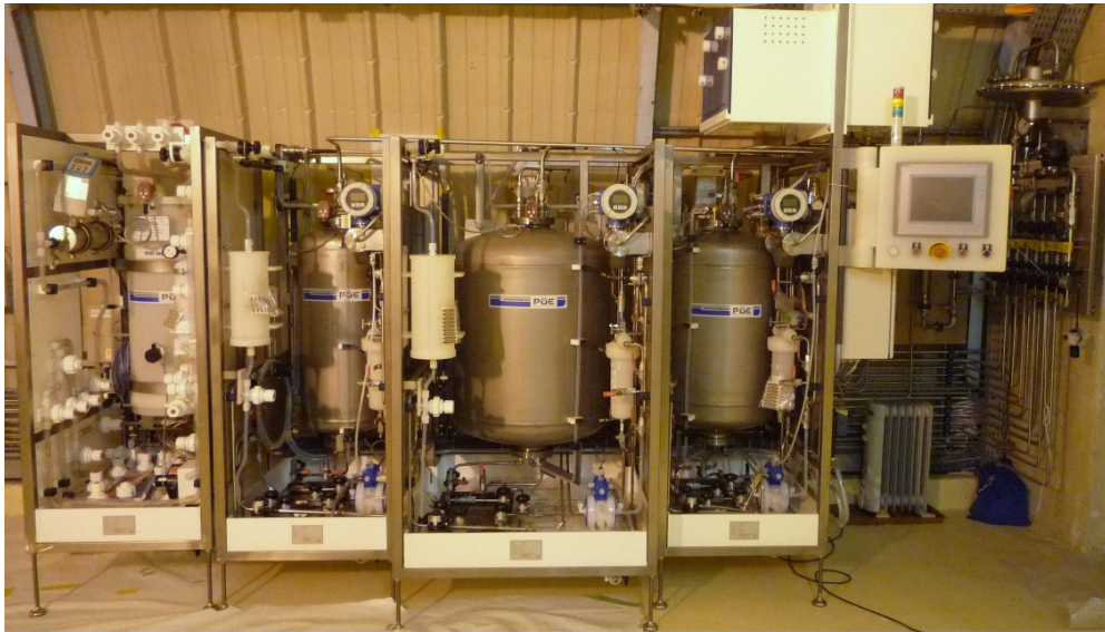
Fig. 9 Detector Fluid Operating System installed in the underground laboratory of the far detector. From left to right are shown: Target, GC, buffer and veto liquid systems; the control unit including touch screen; the over-, underpressure safety and low pressure nitrogen boxes, and one of the gas system manifolds.
