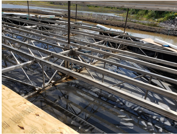
Figure 5: Rows of stringers bolted onto the main support structure. Instrumentation would be attached onto the top of the stringers.
