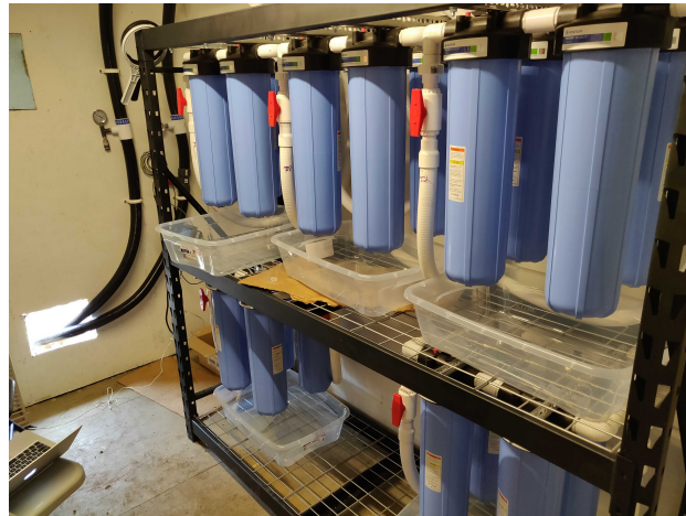
Figure 8: The interior of the water hut showing the filtration plant.
