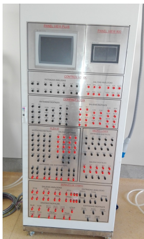
Figure 3: The supervision module
