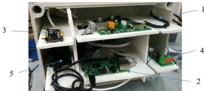
Figure 12: Layout of the electronic unit (1-UHF RFID Reader, 2-Raspberry Pi, 3-LoRa Module, 4-Spray control unit, 5-Power Adapter)
