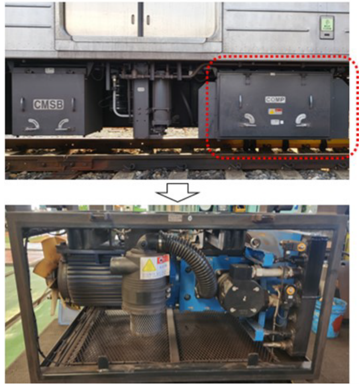
Figure 4: Air compressor of the Electric multiple unit
