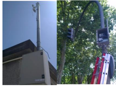
Figure 36: RSUs mounted in the municipality building and in a traffic light
