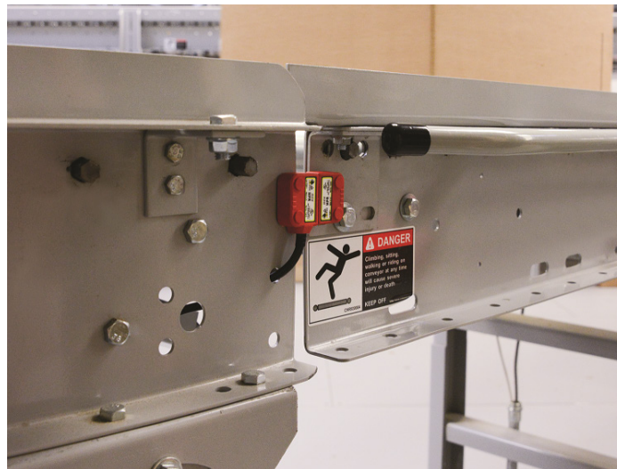
Figure 2: This non-contact safety switch on a conveyor gate tolerates some misalignment while protecting both personnel and conveyor from hazards.
