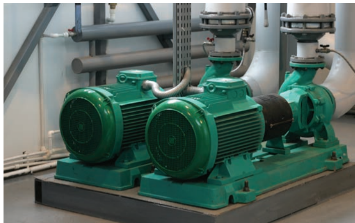
Figure 2: Using VFDs to operate fans and pumps can significantly reduce energy consumption, because they can tailor fan speed to the application. Fan horsepower is proportional to the cube of fan speed, so depending on motor size, energy savings can compensate for the initial VFD purchase price in less than two years.
