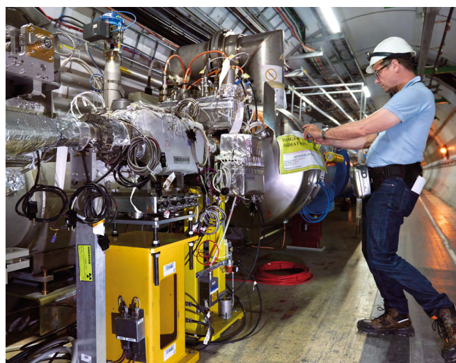
One of the two beam absorbers installed on either side of the LHCb experiment. They are the first definitive components of the HL-LHC to be installed. (CERN-PHOTO-201908-223-4)
