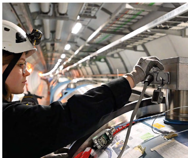
Electrical quality-assurance tests are performed in the LHC in the context of the superconducting-magnet diode-consolidation project. (CERN-HOMEWEB-PHO-2020-048-11)
