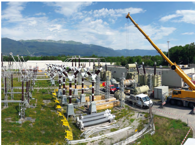
One of the two input substations, on which major maintenance and consolidation work was performed in 2019.
