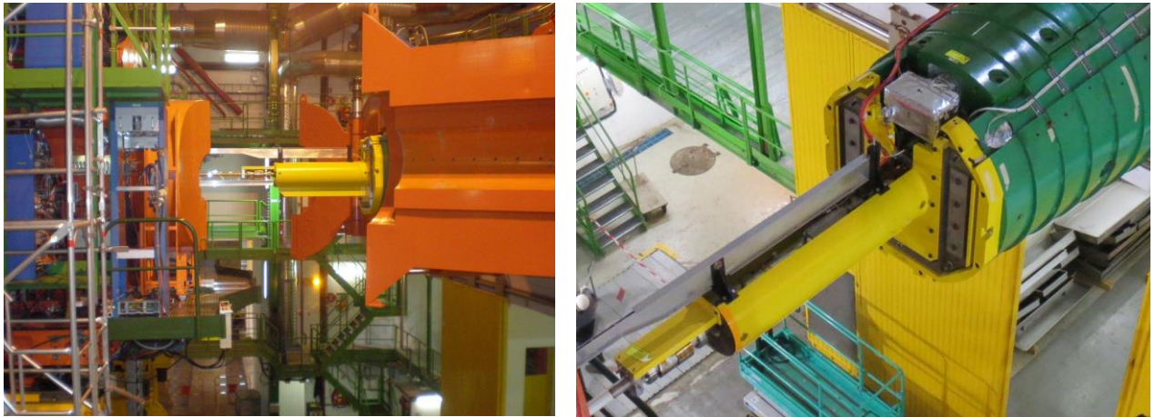
Figure 8-16: Photos showing the CMS forward shielding during access. The small rotating shielding is open, showing the yellow beam pipe support module. Details of the beam pipe support (yellow structure at the tip of the cylindrical tallow support) and the cable tray (Aluminium structure over the yellow support) to be modified are shown on the right picture.
