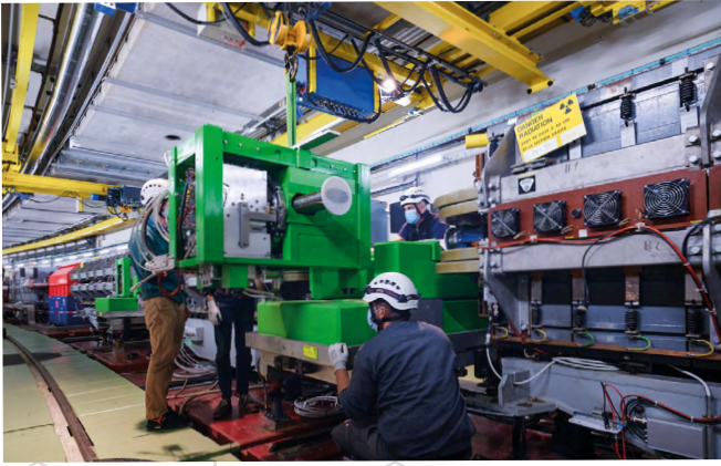
The PS's two new internal beam absorbers, encased in an armoured steel and concrete structure (green), were installed in the accelerator in June.
