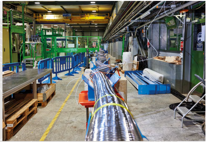
With 54 000 amps transported over a length of 60 metres, this electrical transmission line for the HL-LHC is the most powerful ever built. (CERN-PHOTO-202002-043-5)
