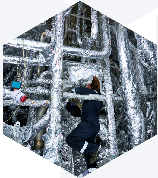
At Point 4, the cold box located on the surface measures around 6 metres in length and 3 metres in diameter. All of its components are vacuum-insulated to limit thermal radiation.
