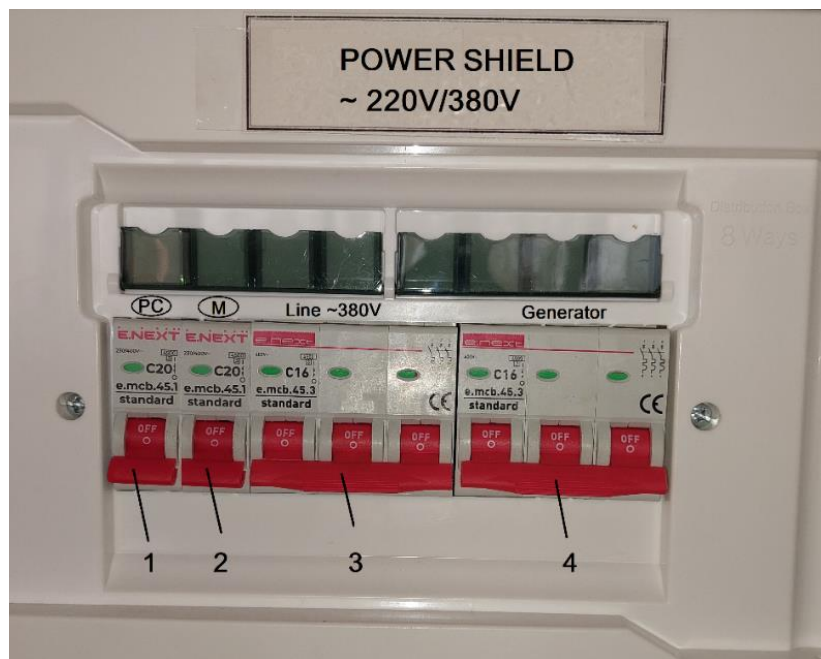
Figure2: Power electrical panel for the laboratory stand power supply: 1 - automatic switch for personal computer powering; 2 - automatic switch for power supply of the load reversing switch drive power supply; 3 - automatic switch of three-phase 380V power line supplied to the load reversing switch; 4 - automatic switch of three-phase 380V generator supplied to the load reversing switch.
