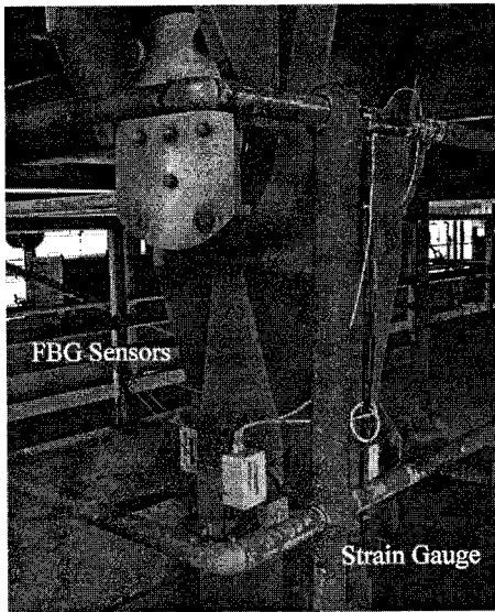
Figure 9 : FBG sensors installed beside an electrical strain gauge on a rocker bearing.
