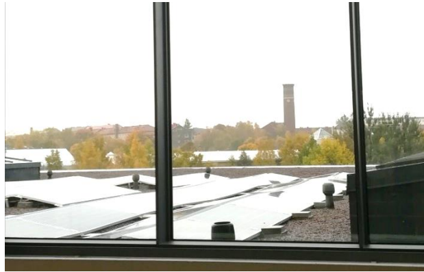
Figure 4. Solar panels, Arcada 2017
