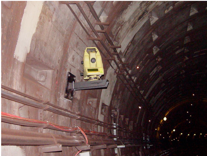
Figure 12 Tunnel monitoring: left total station with bright spots showing reflectors (right) located around tunnel section (below right)
