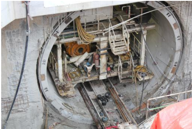
FIG. 2. A constructed tunnel ring at the end of one of the tunnel tubes. Each ring is 1.8 m long and consists of seven concrete segments and one smaller key stone
