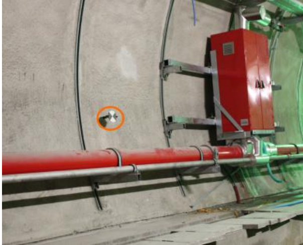
FIG. 8. Black-and-white reference marker (ringed) attached to the bolt in the tunnel surface.
