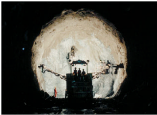
Figure 1. An Atlas Copco drill rig in its natural environment. The vehicle is equipped with rock drills mounted on telescopic booms and is used for drilling holes in the rock face before blasting.
