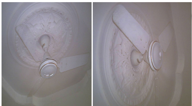
Figure 4 A photograph of different types of ceilings illustrating the stylish gypsum and tongue and groove types of ceiling.
