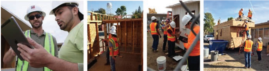
Fig. 4. Students build the tiny solar house with installation details from BIM via tablets.
