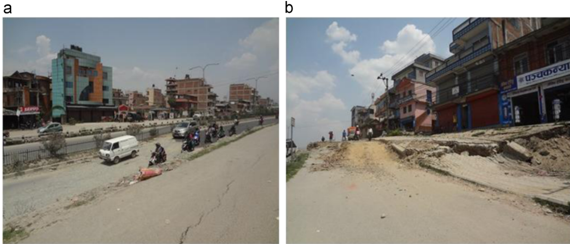
Fig. 25. Slope failure and subsidence (Bhaktapur side). (a) Sinking of the main road and (b) slope failure in the access road.
