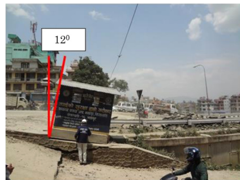
Fig. 24. Slope failure in the Kathmandu side.
