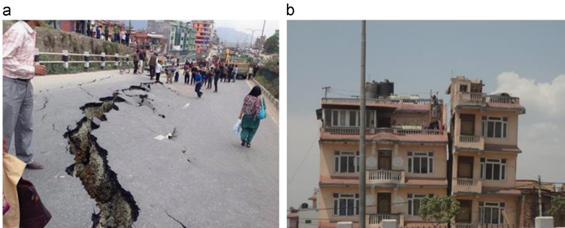
Fig. 26. Access road and building damage (Kathmandu side). (a) Subsidence of the access road and (b) tilted building.
