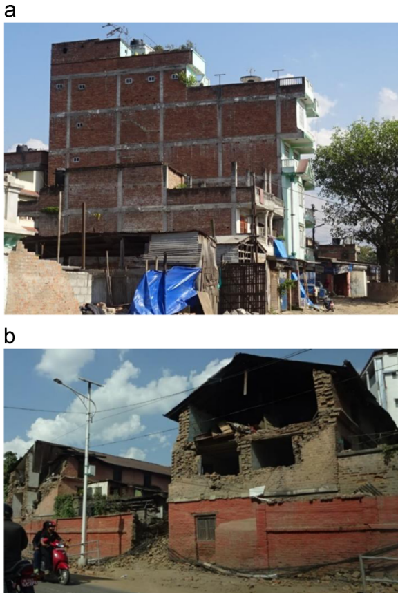
Fig. 12. Typical buildings assessed. (a) six-story RCIW residential building that suffered Grade 1 damage. (b) three-story brick URM houses that suffered Grade 4 damage.
