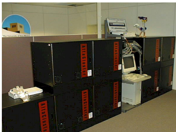
FIGURE 3. Linux prototype on lower-left, and Roadrunner (right). A Myricom dual 8-port SAN Myrinet switch sits on top of the left-most cabinet of the prototype, and four octal 8-port SAN Myrinet switches (not visible) connect Roadrunner. Above Roadrunner's console is a 72-port Foundry Fast Ethernet switch with Gigabit uplinks to the vBNS and Internet. (Image credit: Courtesy of the author.).
