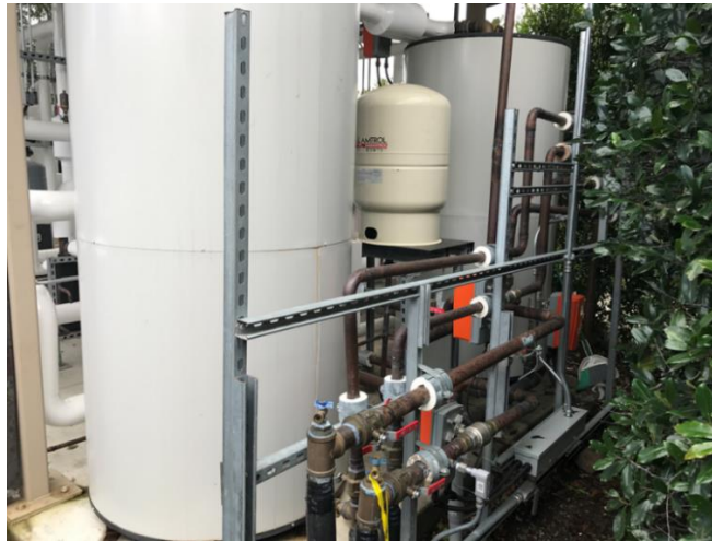
Figure 2-7: Boiler in Stone Edge Farm MES.
