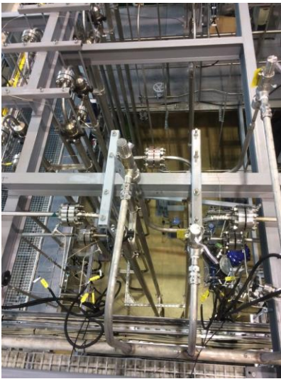
Figure 2: A view from the top to the built sCO 2 loop.
