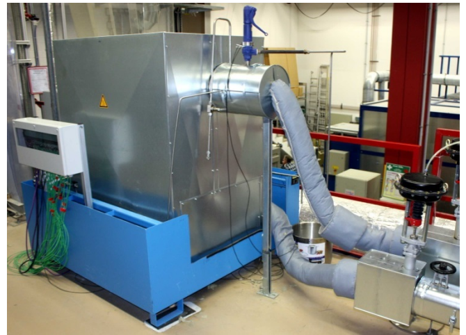
Figure 3: Integration of experimental storage unit in heating and cooling loop.
