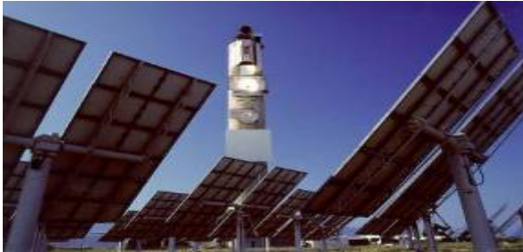
Solar thermal power plants
