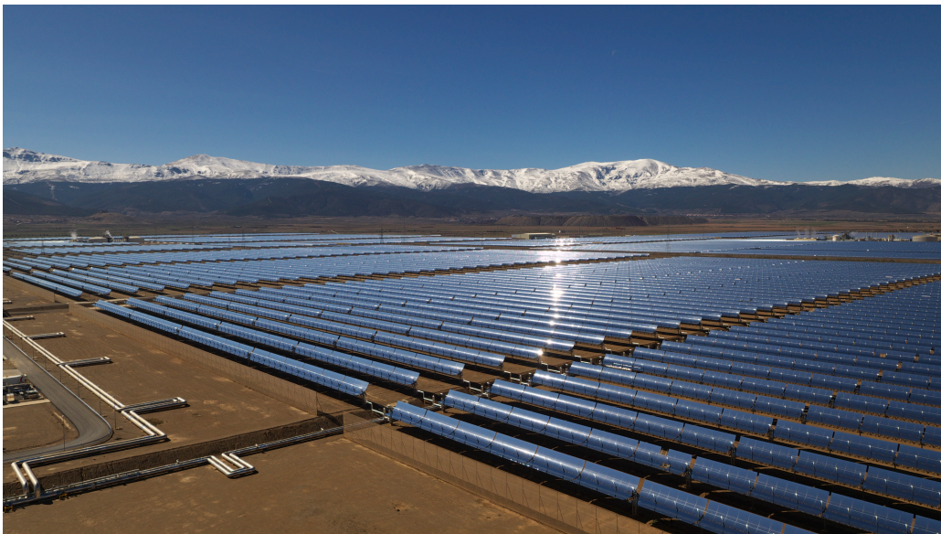
Figure 2.1: CSP plant Andasol III [Source: Marquesado Solar]
