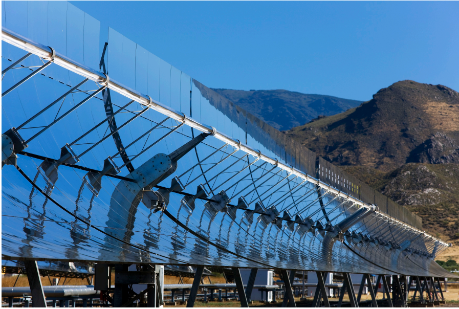
Figure 2.3: Parabolic Trough Collector at the Plataforma Solar de Almería (PSA). Owner and operator of PSA is the Research Center CIEMAT. [Source: DLR/Markus-Steuer.de.]
