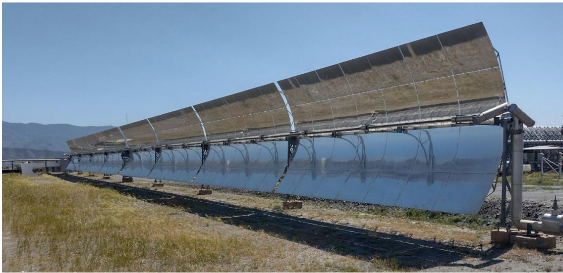
Figure 2.2, Solar collector at Plataforma Solar de Almería (owned by CIEMAT)
