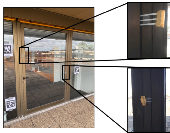
(b) Constructed leaks in the window
