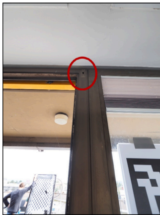
(a) Existing leak in the window
