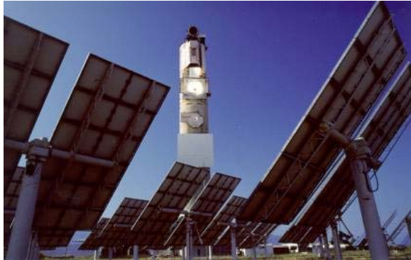
Solar thermal power plants
