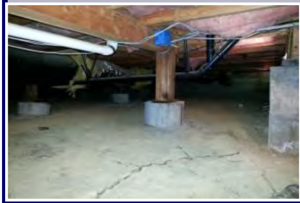
Rupture through piers
