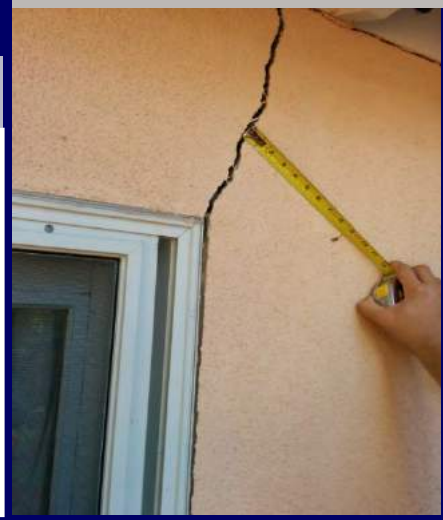
Damage to structure
